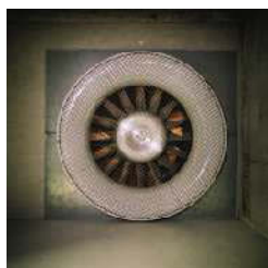
Application de ventilation
